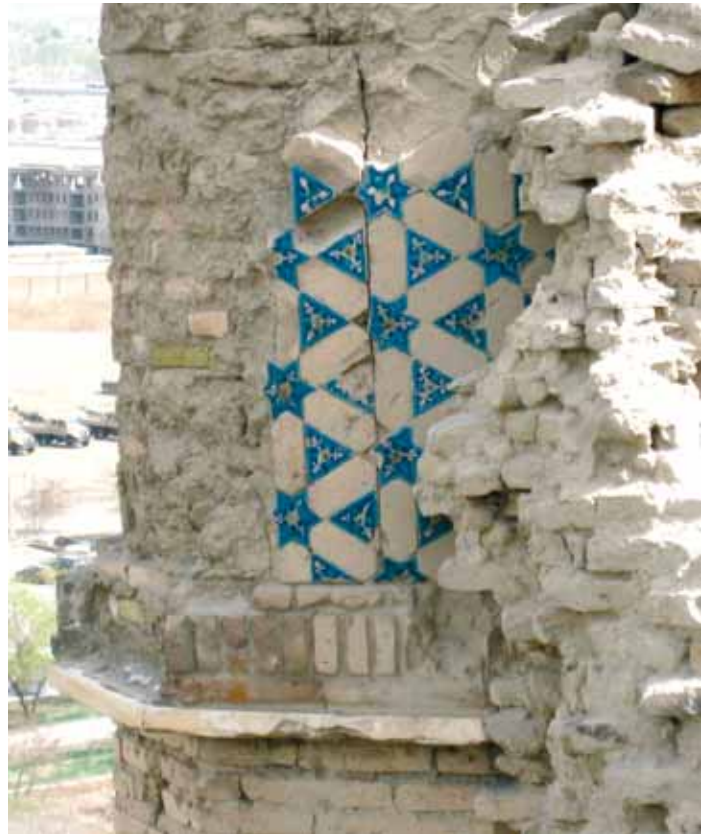
Figure 18. Remains of tiling above a string-course on the upper part of the platform in Figure 17. [J.Leslie.]
