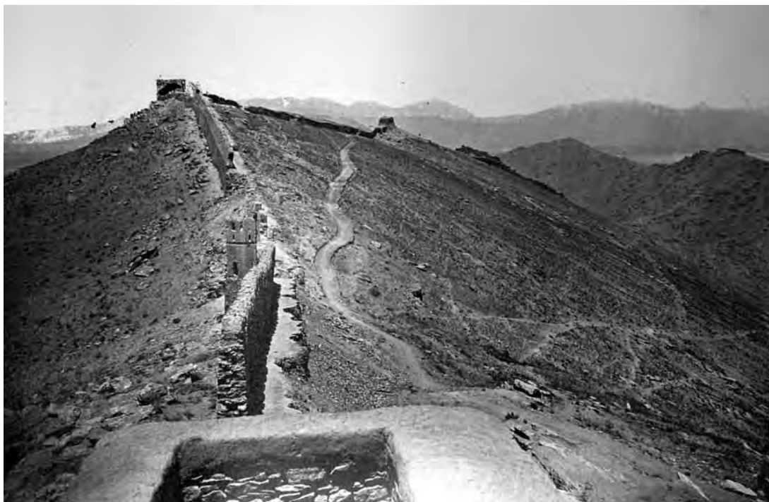
Figure 52. Posts which were strengthened along Sher Dawza walls in 1880. The road built at this time lies along the right (north) side. [Bengal Sappers & Miners; Institution of RE]
