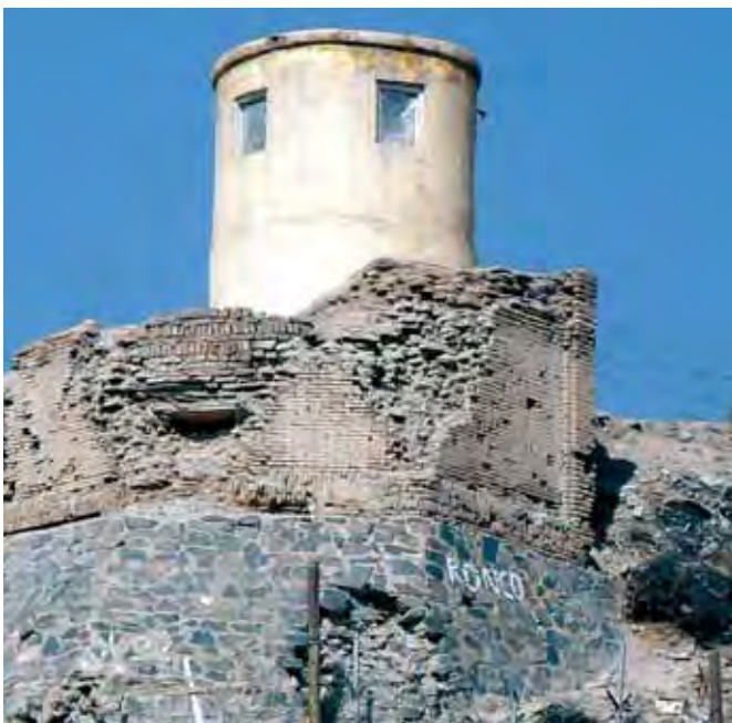
Figure 16. The base of the south tower of the Mughal period Darwaza Kashi ; the only bit of the gateway still standing. This part may have been tiled or the tiling might have been on an upper level, with this as plain blind-arcading. The quality of the brickwork is apparent. The tower on the top is modern. [ J.Grindle. ]
